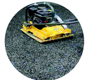
Laying and compaction of leveling layer 30-50 mm - Recommended fraction size of stones 4-8, 8-16 mm
