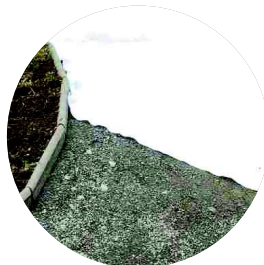
Installation of geotextile - 200 g/m 2 - At least 30 cm overlap of joints is required
