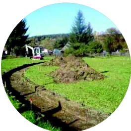
Subsoil preparation Excavation with suitable depth, the depth of the trench according to TOPSTONE normogram
